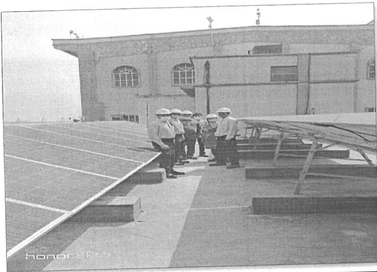
Solar PV Plant at Service Building
